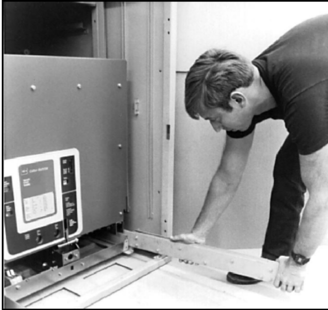
Figure 4-3 Engaging Extension Rails in Drawout Circuit Breaker Compartment
